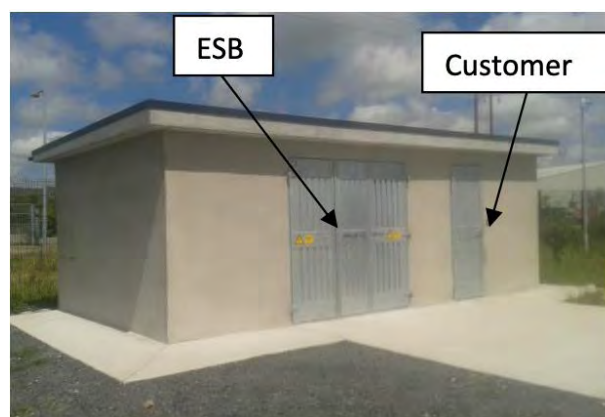
Figure 5-64 Example of MV substation
