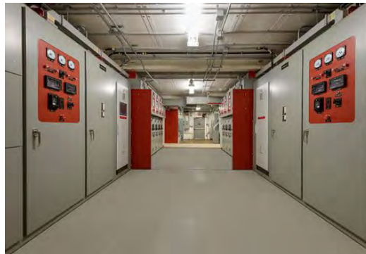
Figure 5-61 Substation switchgear installed
