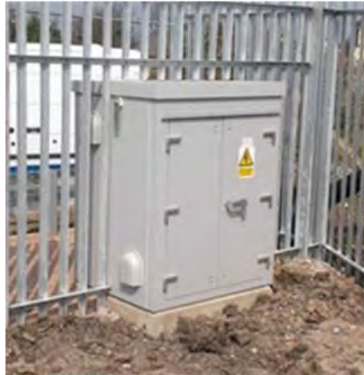
Figure 5-67 Double sided DNO/distribution cubicle
