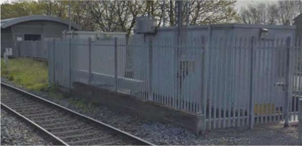
Figure 4-22 Example of typical Telecom Equipment Building
