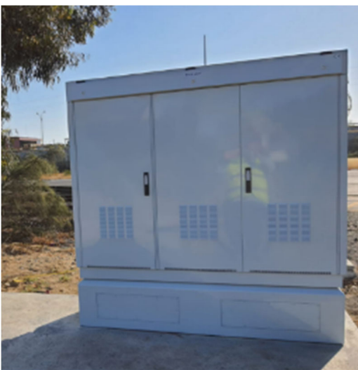
Figure 4-20 Typical Object Controller Cabinet (OBJ)
