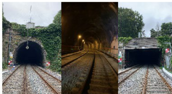
Northern and Southern Portals to the Phoenix Park Tunnel and view of inside tunnel
