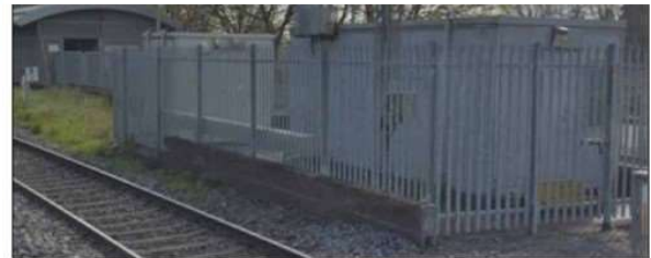
Typical Equipment Cabin
