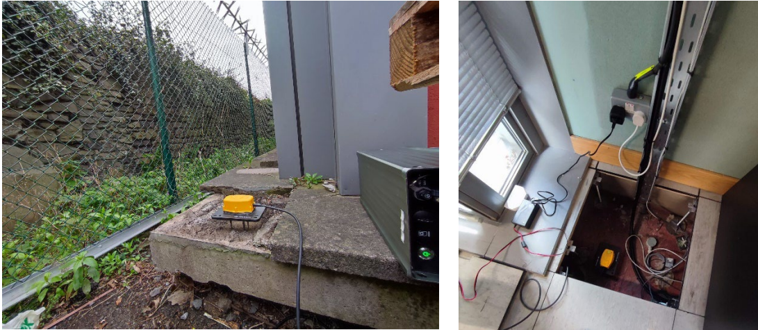
Figure A14-2 Con Colbert House Installation (External (left) and Server Room (right)).
