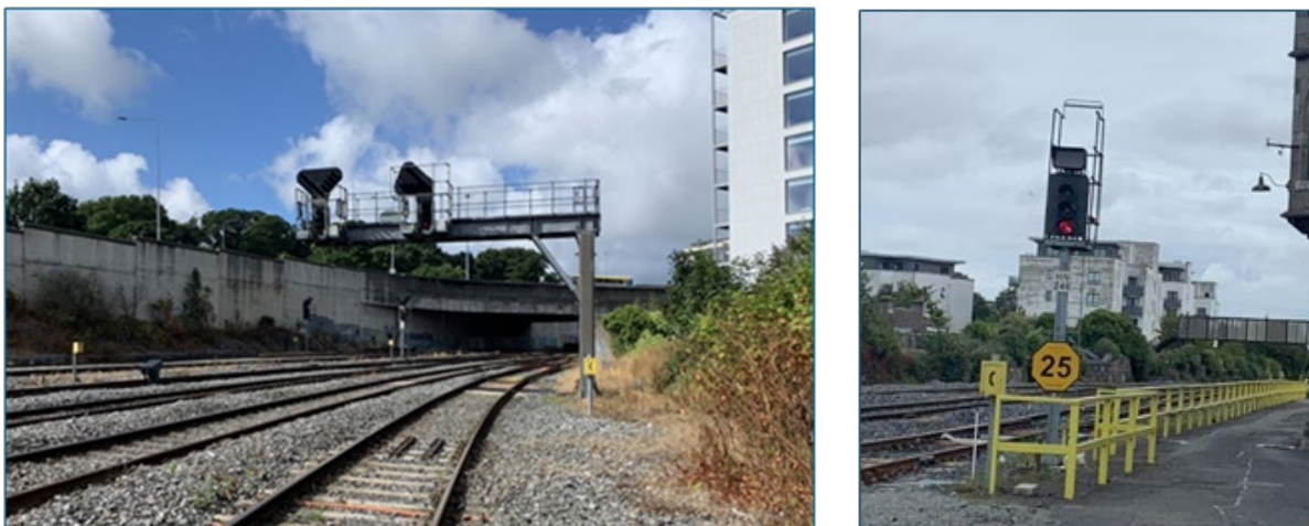
Figure 2-2 Typical Existing Signalling Infrastructure
