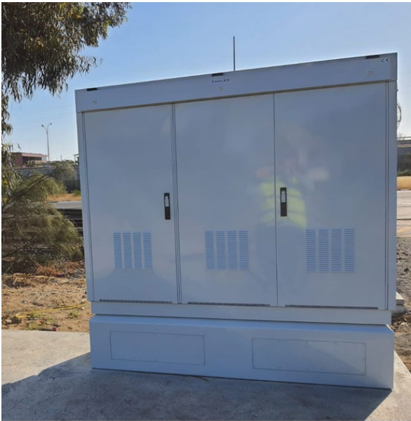
Figure 2-3 Typical Object Controller Cabinet (OBJ)
