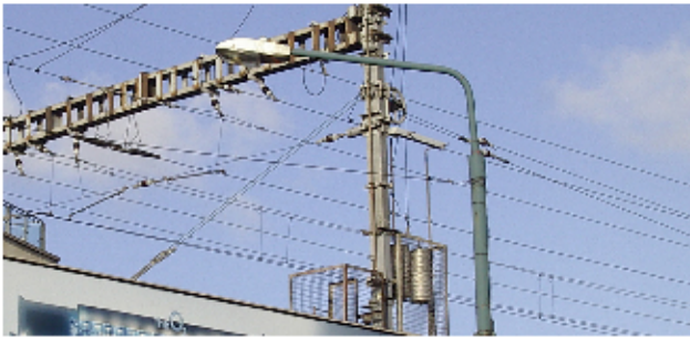
Figure 9. Existing 1500VDC OHLE with gantry on DART network
