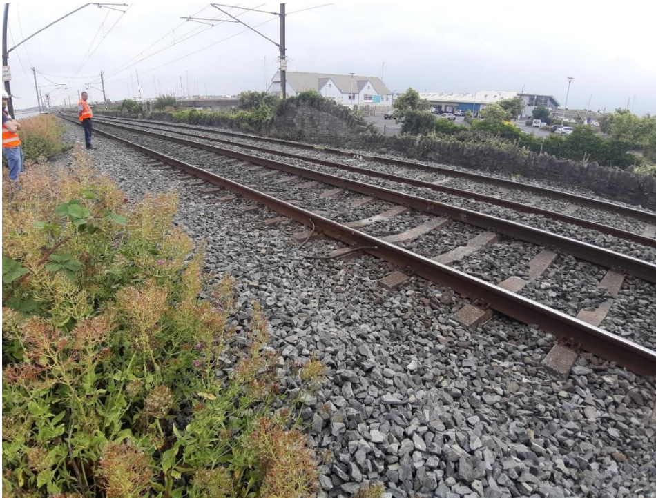
Figure 2-4: Photograph of the mainline North of Malahide Station with Malahide Marina in the background (source: Arup)
