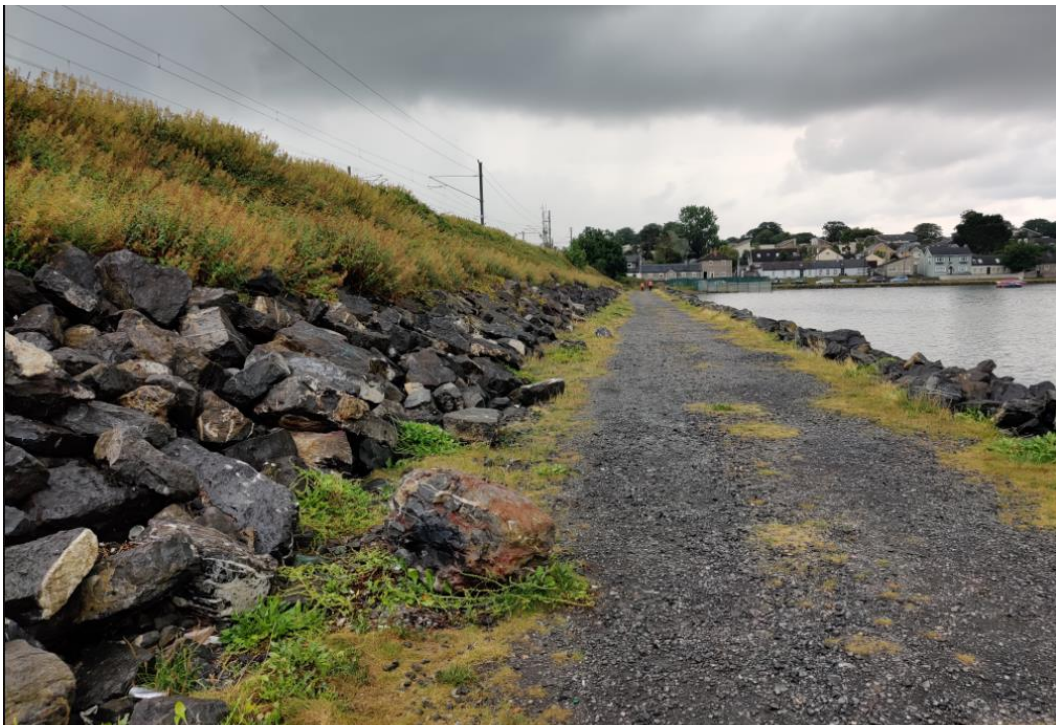
Figure 2-15: View south towards Malahide along the access track on the west of the causeway (source: Arup)
