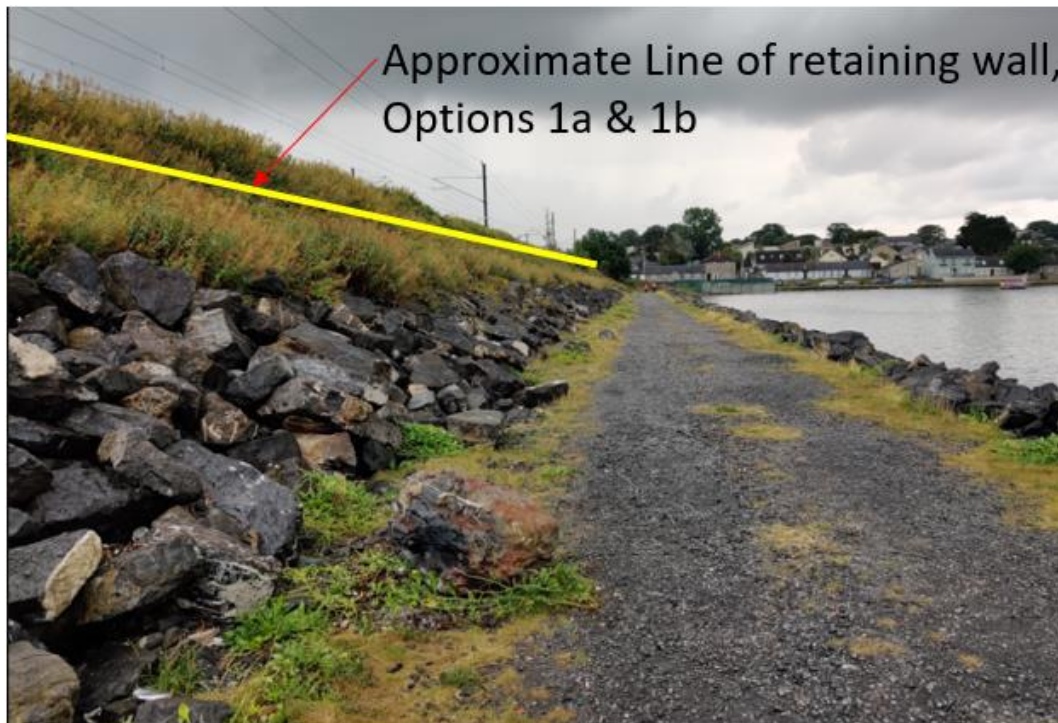
Figure 5-19: Approximate position of Options 1A and 1B retaining wall on west of the embankment (source: Arup)
