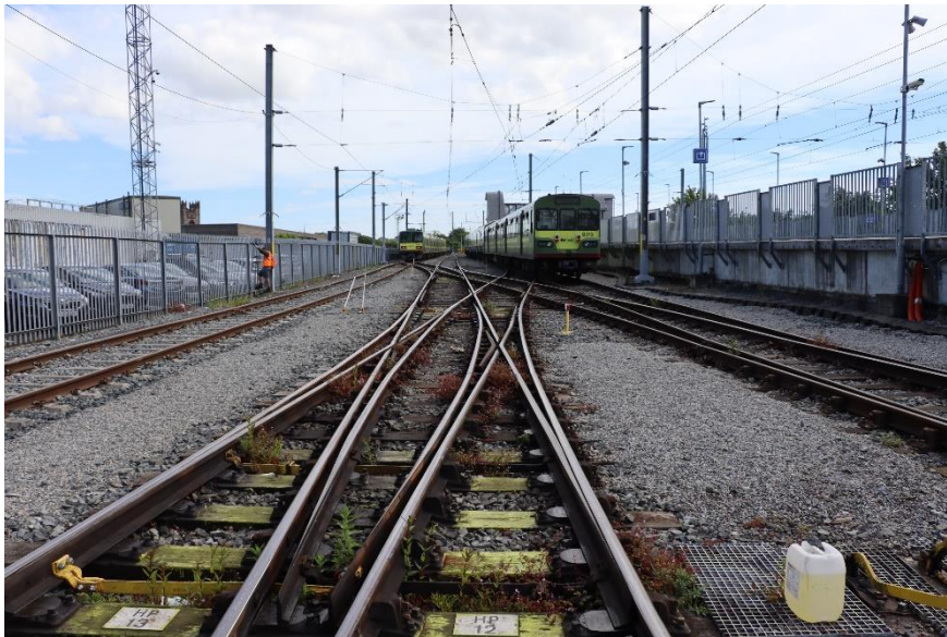
Figure 5-2: A typical OHLE in a densely configured track area
