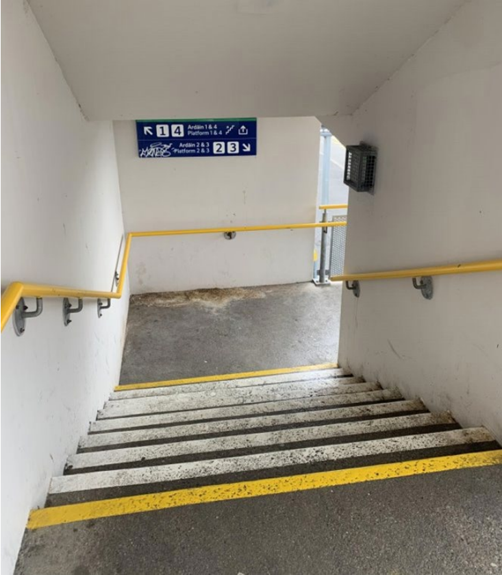
Photo of existing stairs demonstrating the poor visibility
