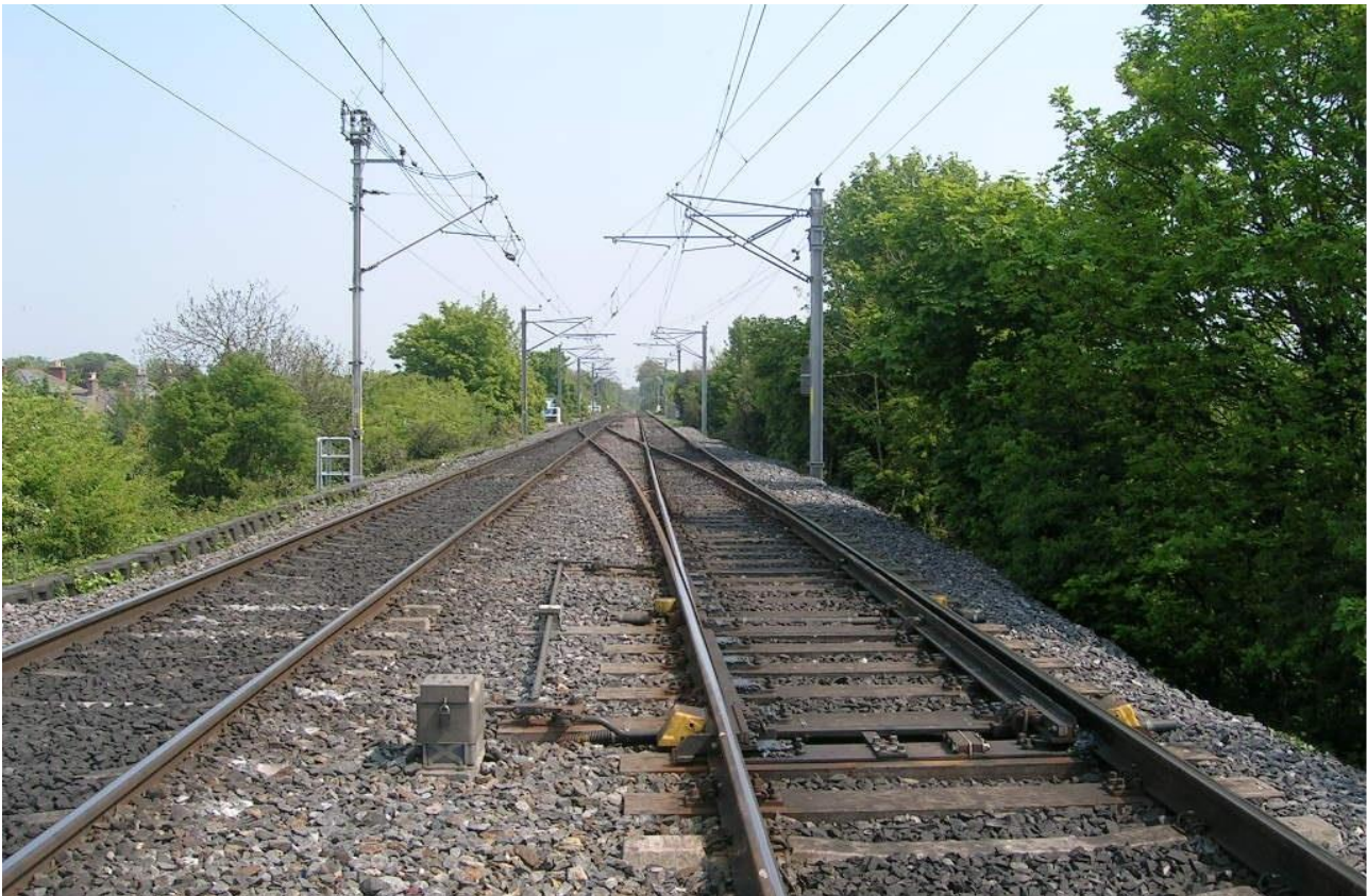
Figure 3-1: An example of OHLE on an existing line
