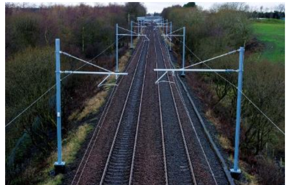
Figure ES-3 OHLE Infrastructure
