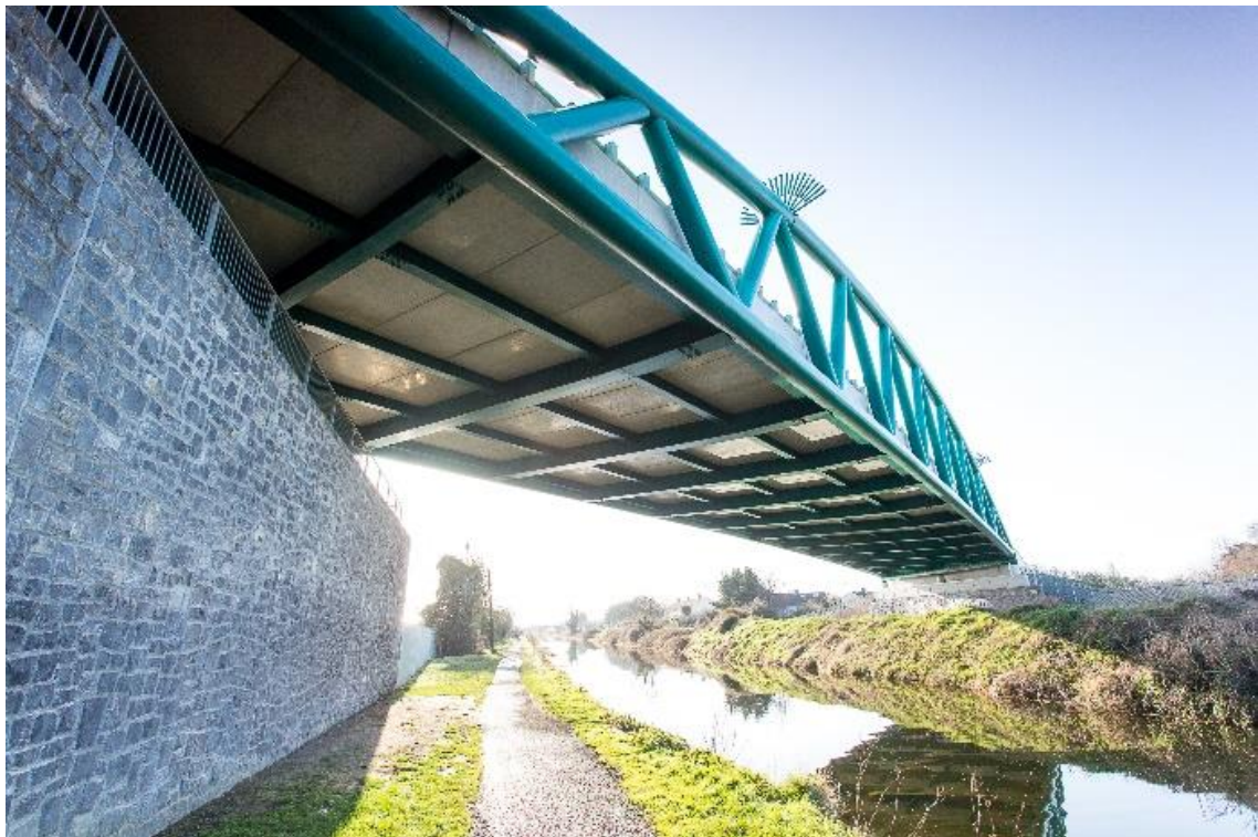
Figure 2-4 View of the canal and towpath beneath the Ratoath Road (Reilly's) bridge
