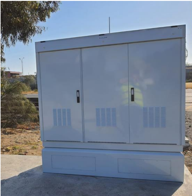
Figure 7-5 Typical Object Controller Cabinet
