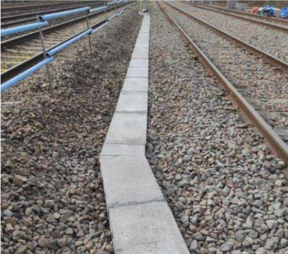
Figure 5-12 Example of Concrete Cable Troughing
